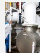
Ballast Water Treatment
